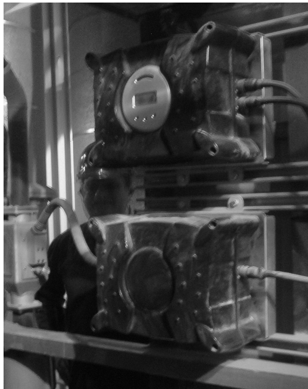
Figure 3: A Blue Cube MQi installed in a dry mineral stream
