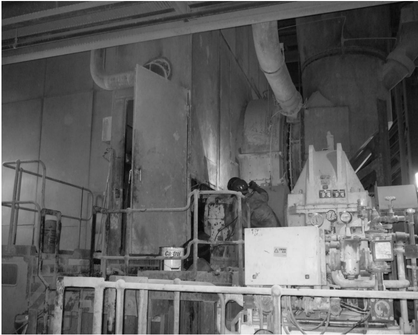
Picture 2: Typical installation on a 1800 kW Ball Mill (courtesy of Kendal Power Station, South Africa)
