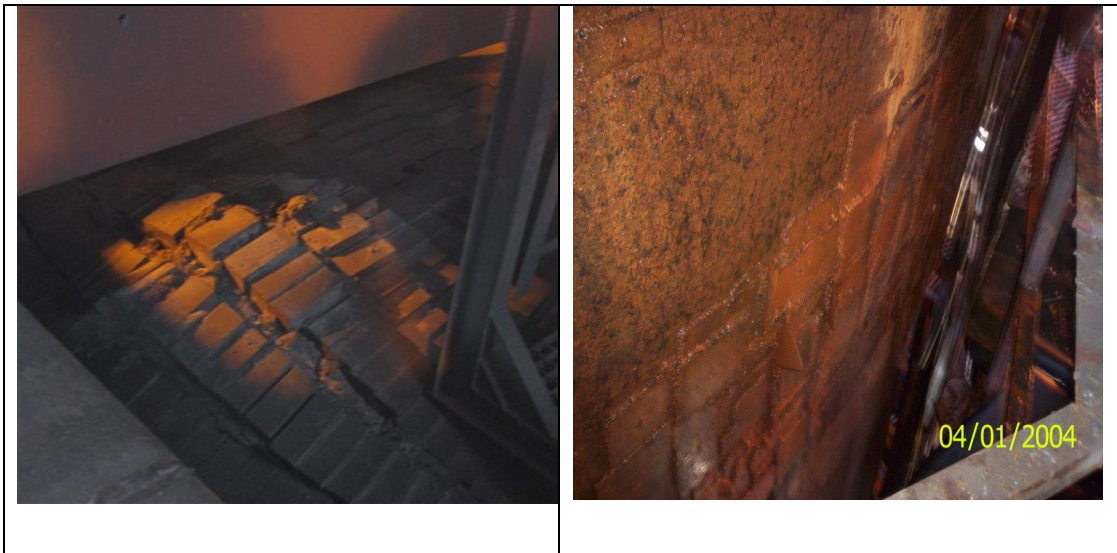
Figure 3. Reaction shaft roof damage
